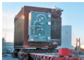
Sturgeon Refinery - Canada (3 x 35 MWe)
