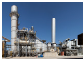
Granada - Spain (1 x 45 MWe)
